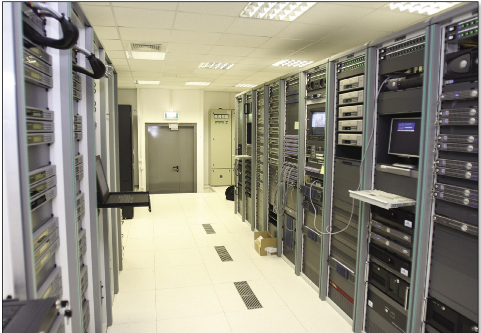
The central apparatus room houses Harmonic encoders and multiplexers, as well as the playout channels.
